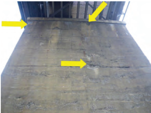
Pier 2 pier wall, south face - Map/vertical cracks with moisture throughout, delamination along pier cap and scattered delaminations, spalls, and scaling.
