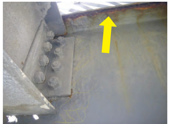
Span 4 - Floor beam web and top flange section loss adjacent to/above stringer connection.
