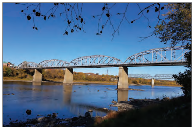
The existing International Bridge from the bank of the Saint John River on the Madawaska side looking northeast.
