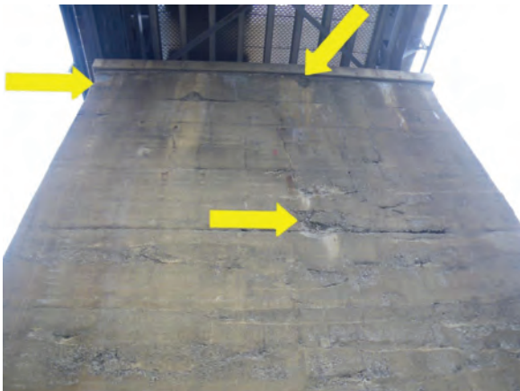
Pier 2 pier wall, south face - Map/vertical cracks with moisture throughout, delamination along pier cap and scattered delaminations, spalls, and scaling.
