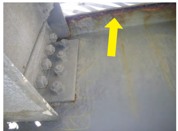
Span 4 - Floor beam web and top flange section loss adjacent to/above stringer connection.
