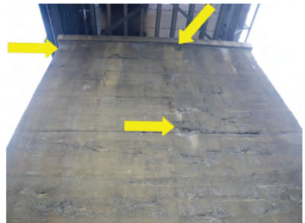
Pier 2 pier wall, south face - Map/vertical cracks with moisture throughout, delamination along pier cap and scattered delaminations, spalls, and scaling.
