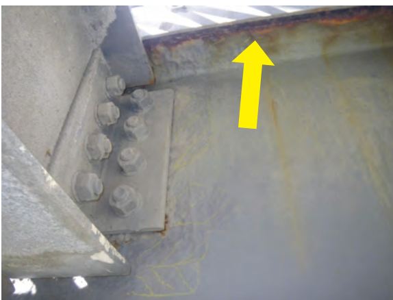
Span 4 - Floor beam web and top flange section loss adjacent to/above stringer connection.
