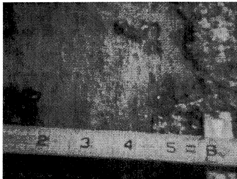
Photo # 2 South Pier, Station 10, elevation mean low water, surface cleaned for steel thickness reading
