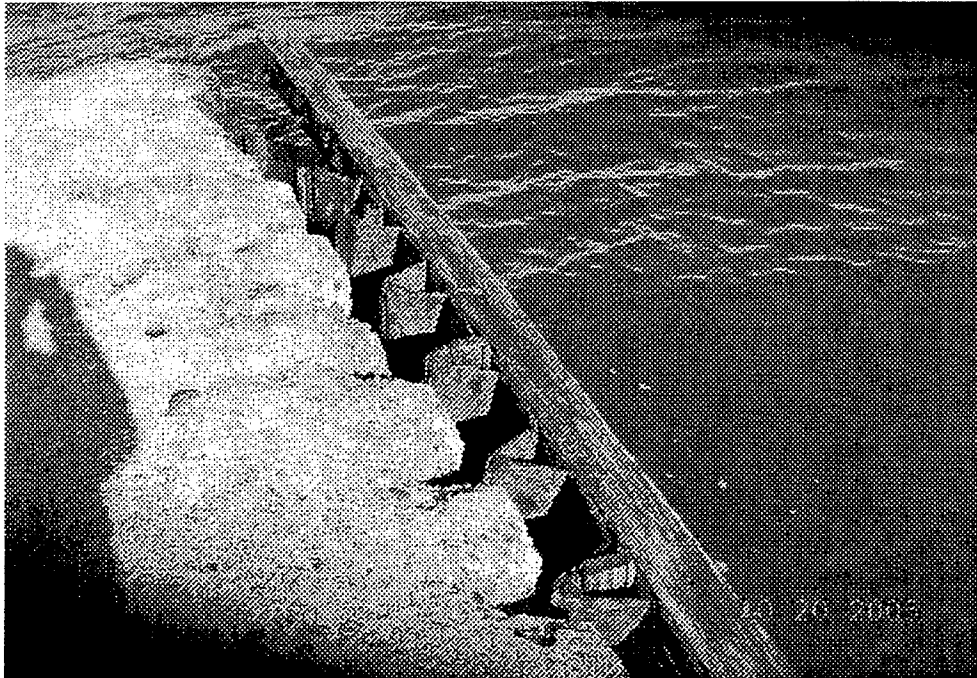
Photo # 8, North Pier, Sheet pile on South east face is separated
