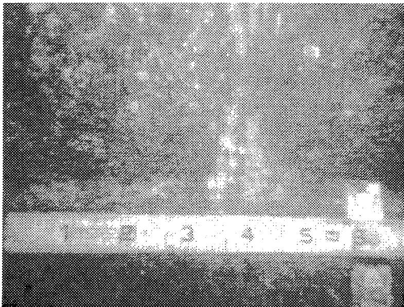
Photo # 6 Center Pier, typical granite block joint open 2 1/2"
