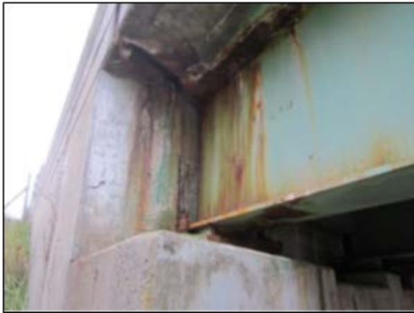
I-95 NB/SB over Webb Road Bridges – Poor Deck End and Backwall Condition due to Failed Deck Joint
