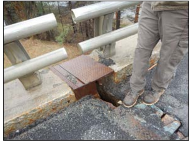
Vaughan Daggett Memorial Bridges- Condition of deck joint at north abutment and sub-standard bridge rail
