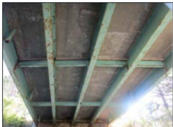
Route 155/I-95 Bridge – Scattered Cracking, Efflorescent Staining, and Delamination of Underside of Deck
