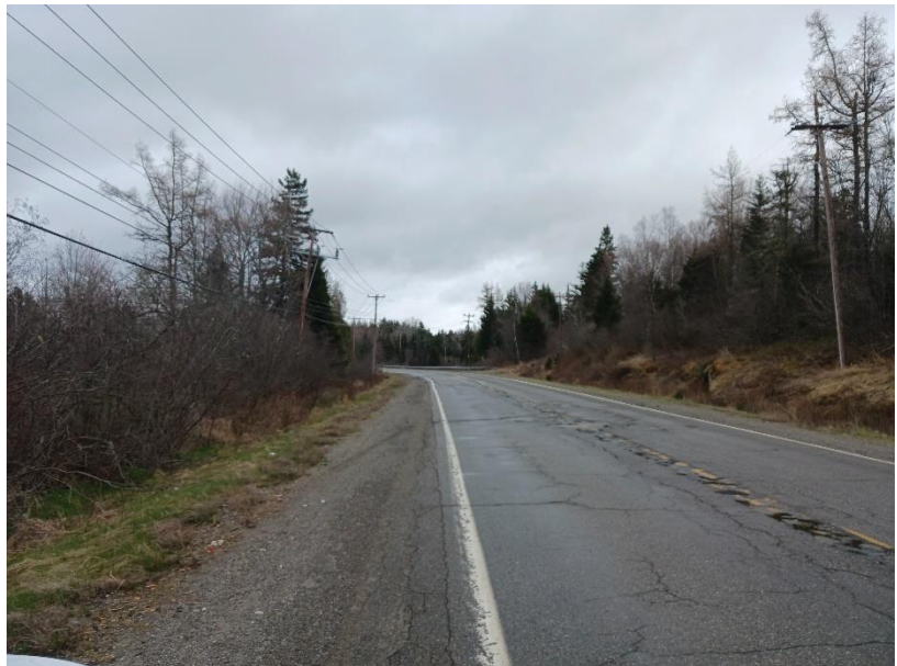
Deteriorating road condition and unpaved shoulders along US 1. Photo courtesy MaineDOT
