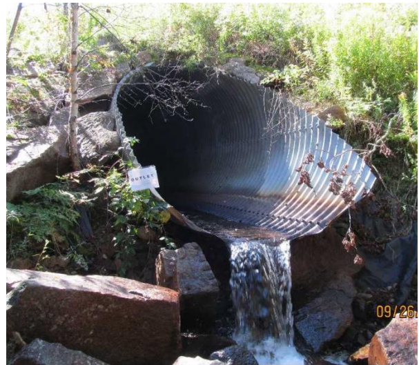
Large Culvert 4367 – Fish Passage Barrier
