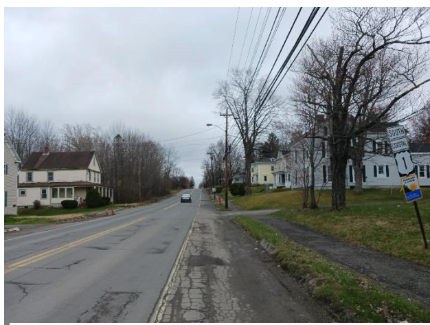
Deteriorating Shoulder along US 1. Photo courtesy MaineDOT.
