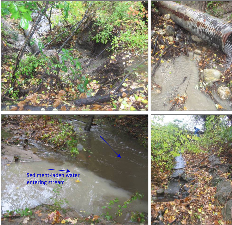
Site 1 Photos, continued: View from above of failed bank surrounding the culverts (upper left); sediment-laden water flows under culverts (upper right); sediment laden water entering stream (bottom left); concrete sluiceway draining McDonalds lot (bottom right).
