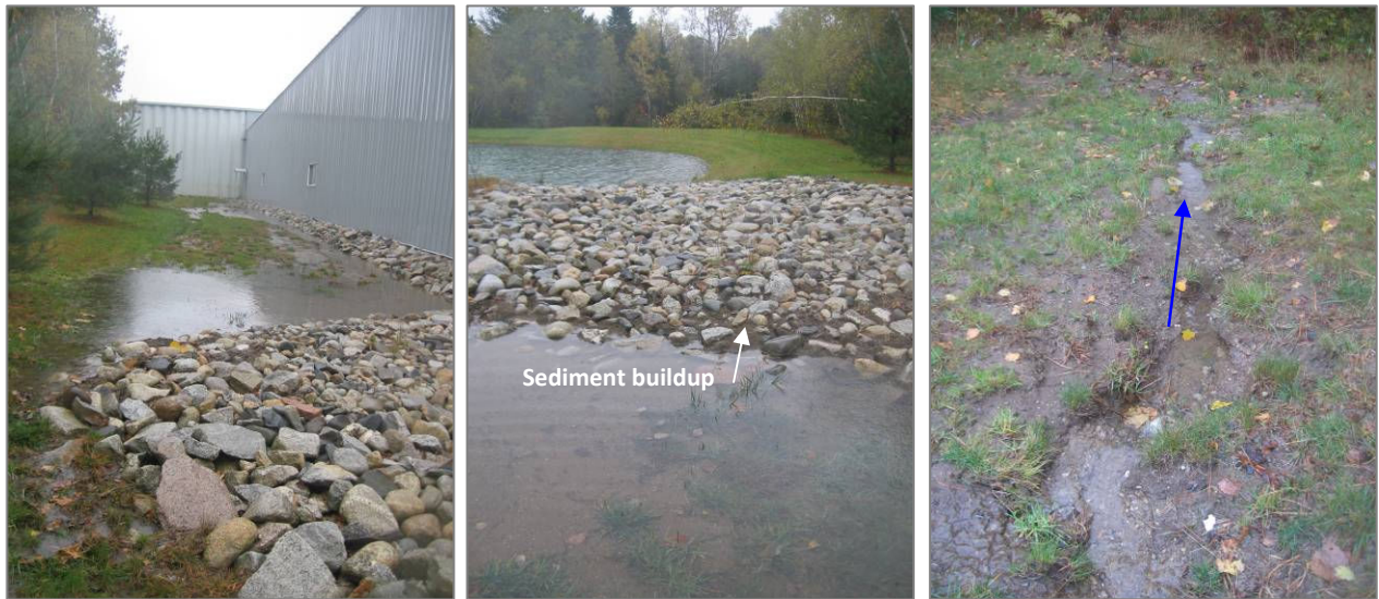
Site 5A Photos: Stormwater runoff pools behind the Owen's Corning building (left); water pools at the detention basin inlet (middle); excess runoff results in an eroding channel (right).
