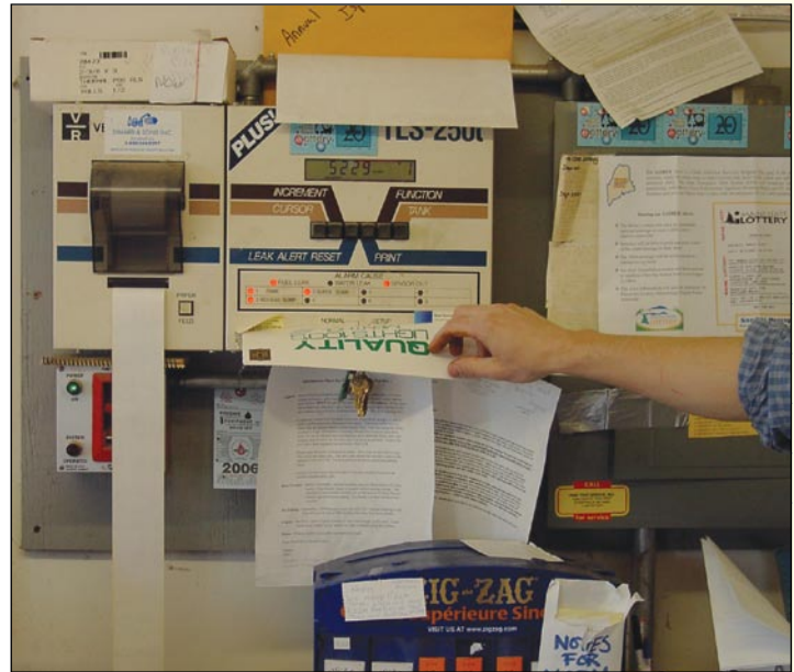
Do not cover up or ignore alarms. In this photo, a piece of paper was taped over the alarm lights so they could not be seen. This is NOT the proper response to an alarm!
