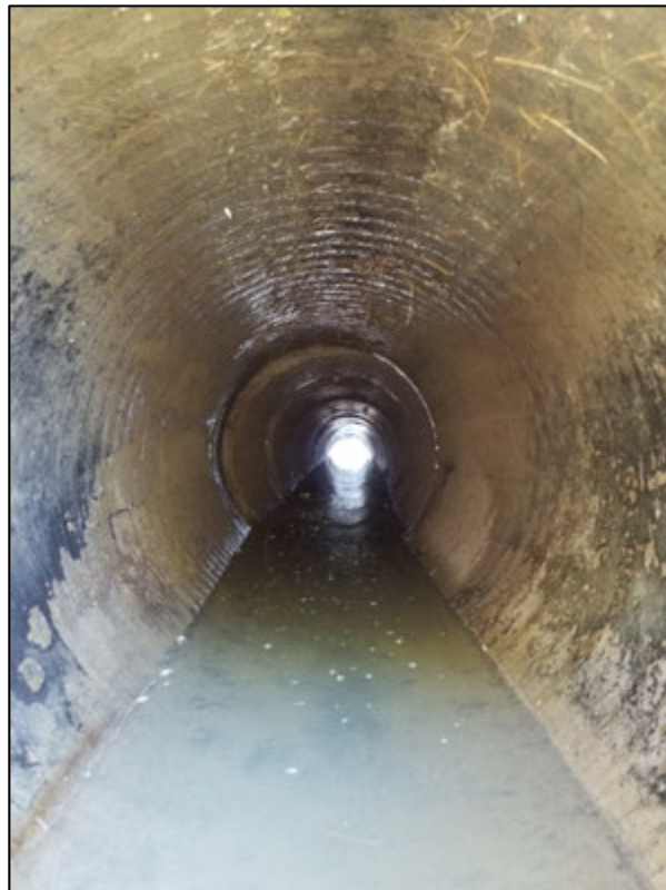
Photo 6: Interior of Culvert. Sections Have Shifted (Photo Taken 11/11/2020)
