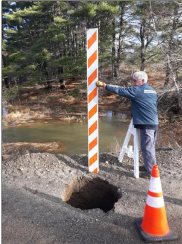
Photo 7: Sinkhole Formed Along Culvert Crossing (Photo Taken on 8/10/2020)
