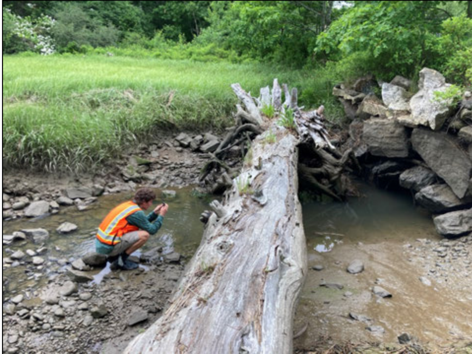
Photo 5: Headwall Collapse at Outlet (Photo Taken 11/11/2020)
