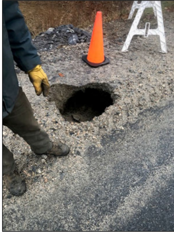
Photo 9: Sinkhole Formed Along Culvert Crossing (Photo Taken on 8/10/2020)
