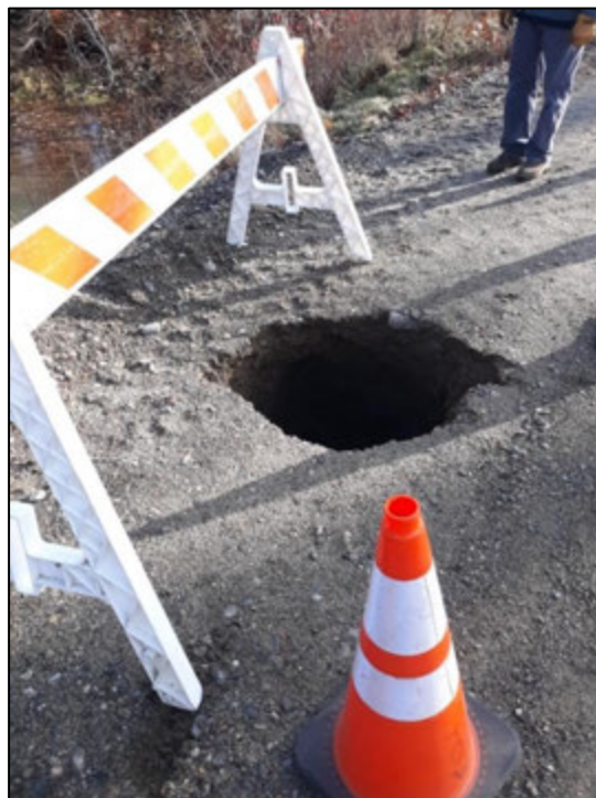
Photo 8: Sinkhole Formed Along Culvert Crossing (Photo Taken on 8/10/2020)
