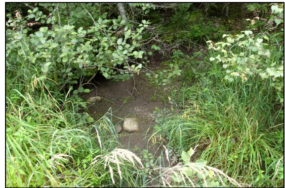
Sedimentation into wetland at outlet of culvert.
