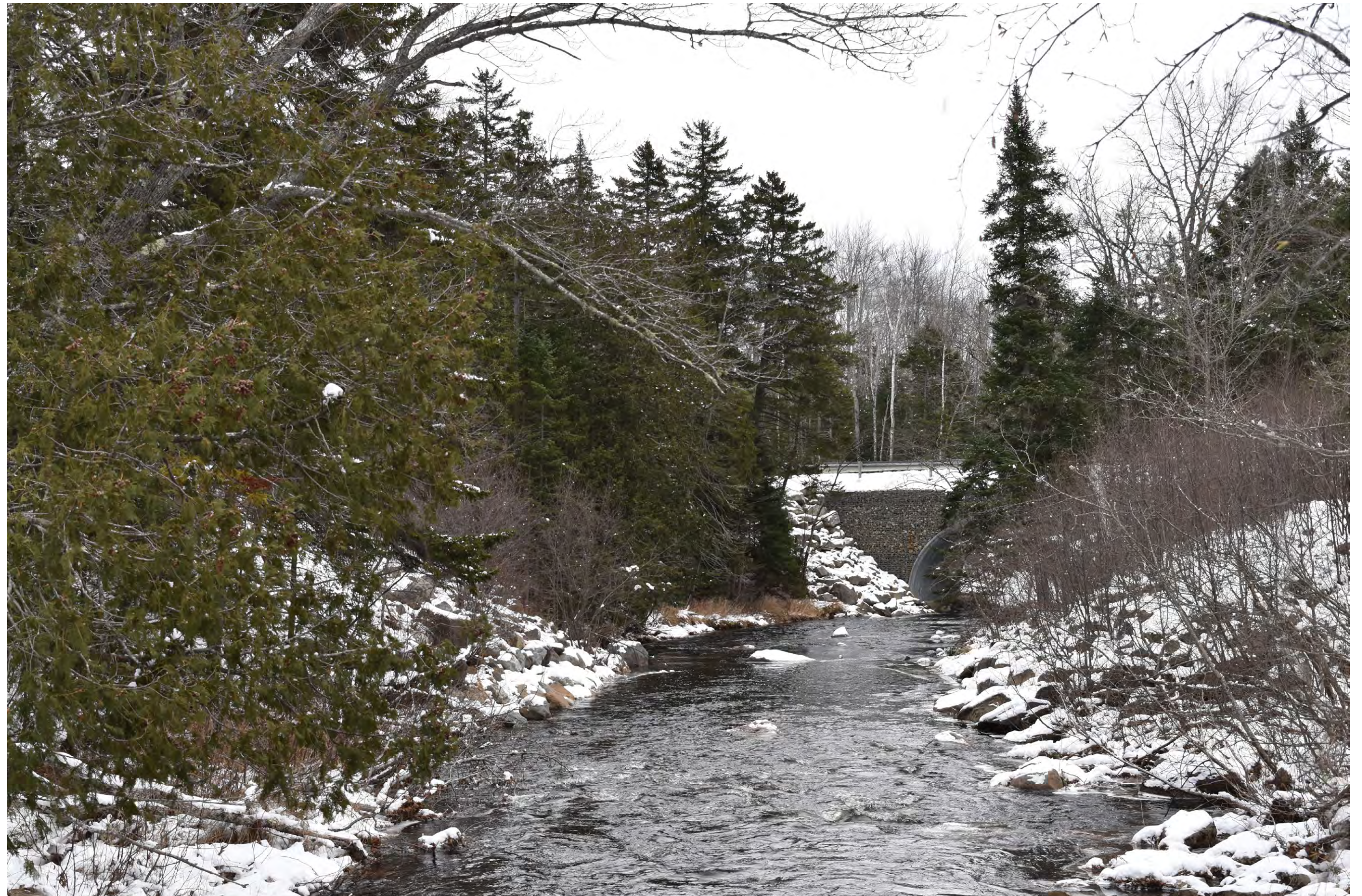
Existing Conditions: Normal view looking east on the ITS 87 bridge over Cold Stream toward the Capital Road bridge, within the Cold Stream Forest parcel in Johnson Mountain Twp.
