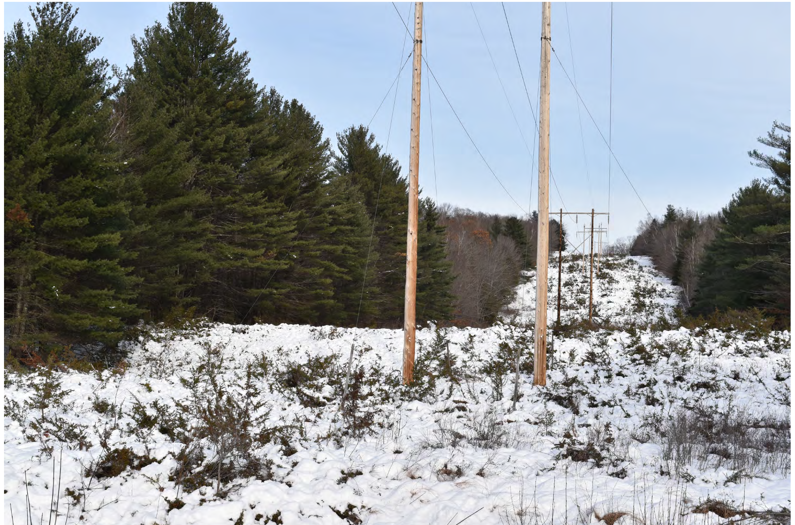
Existing Conditions: Normal view looking northeast toward the existing 115 kV transmission line corridor from Route 201 in Moscow.
