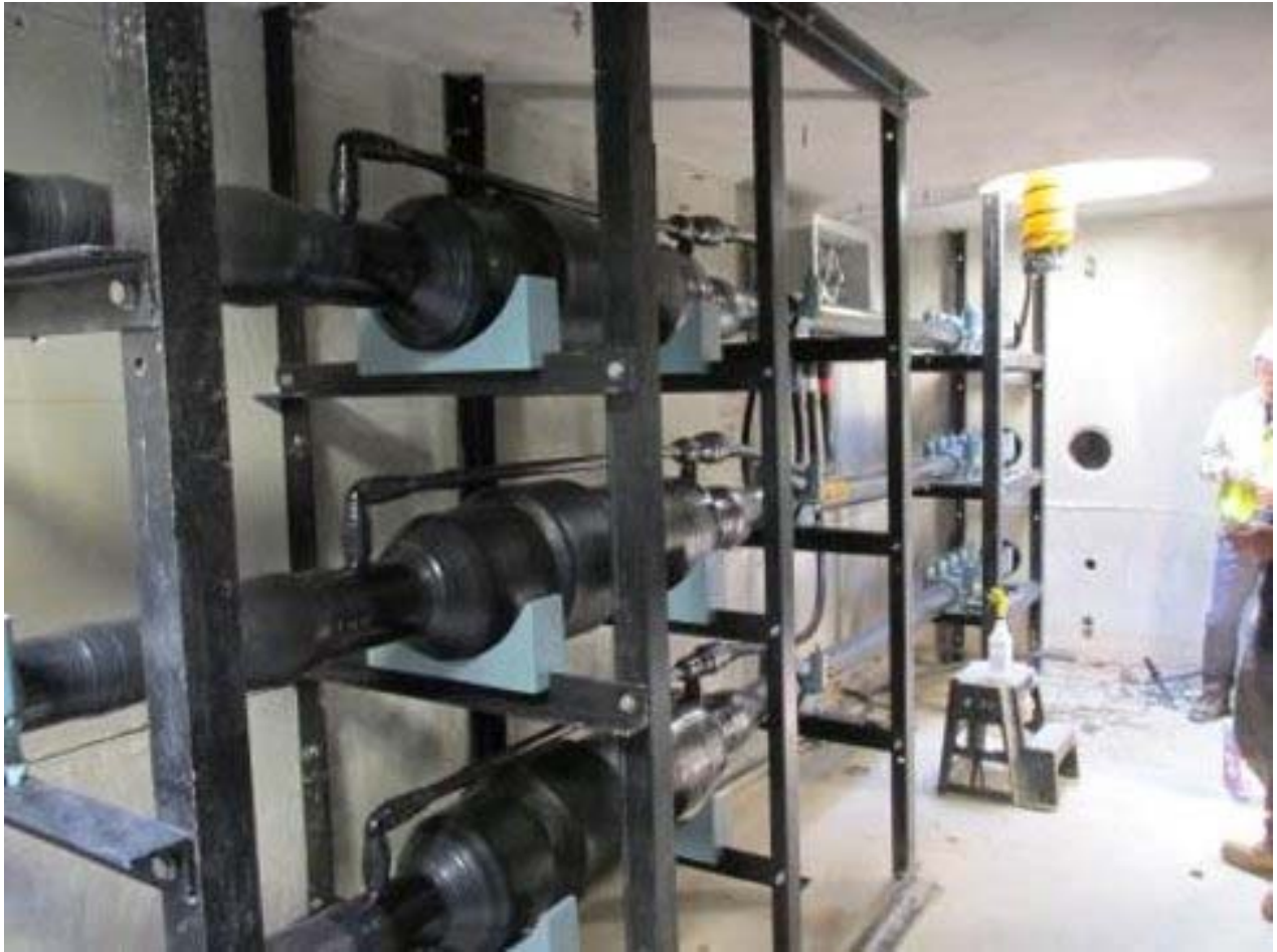
Figure 15 - Cable Joints in Vault
