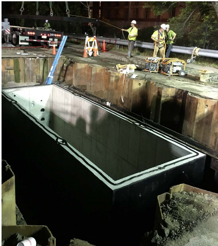
Figure 4- 115kV Splicing Vault
