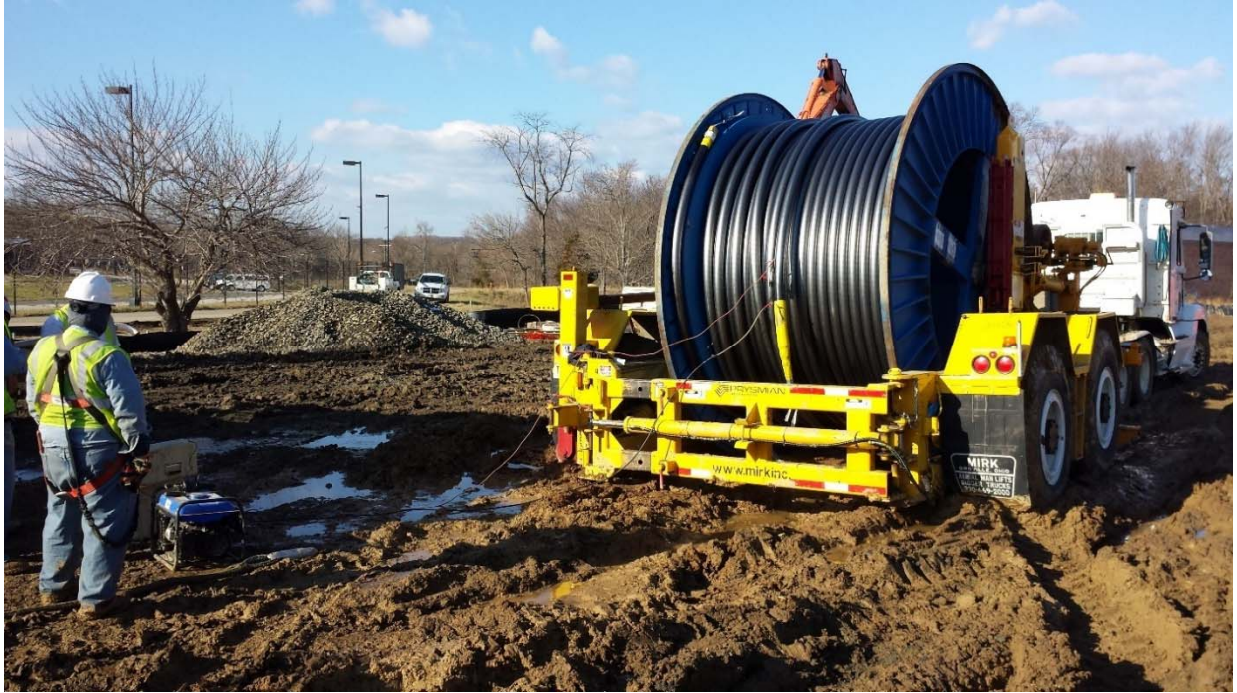
Figure 11 - Cable Reel Trailer
