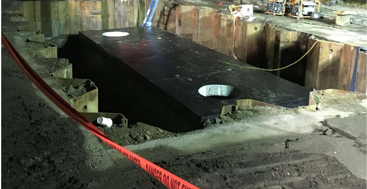
Figure 5- 115kV Splicing Vault
