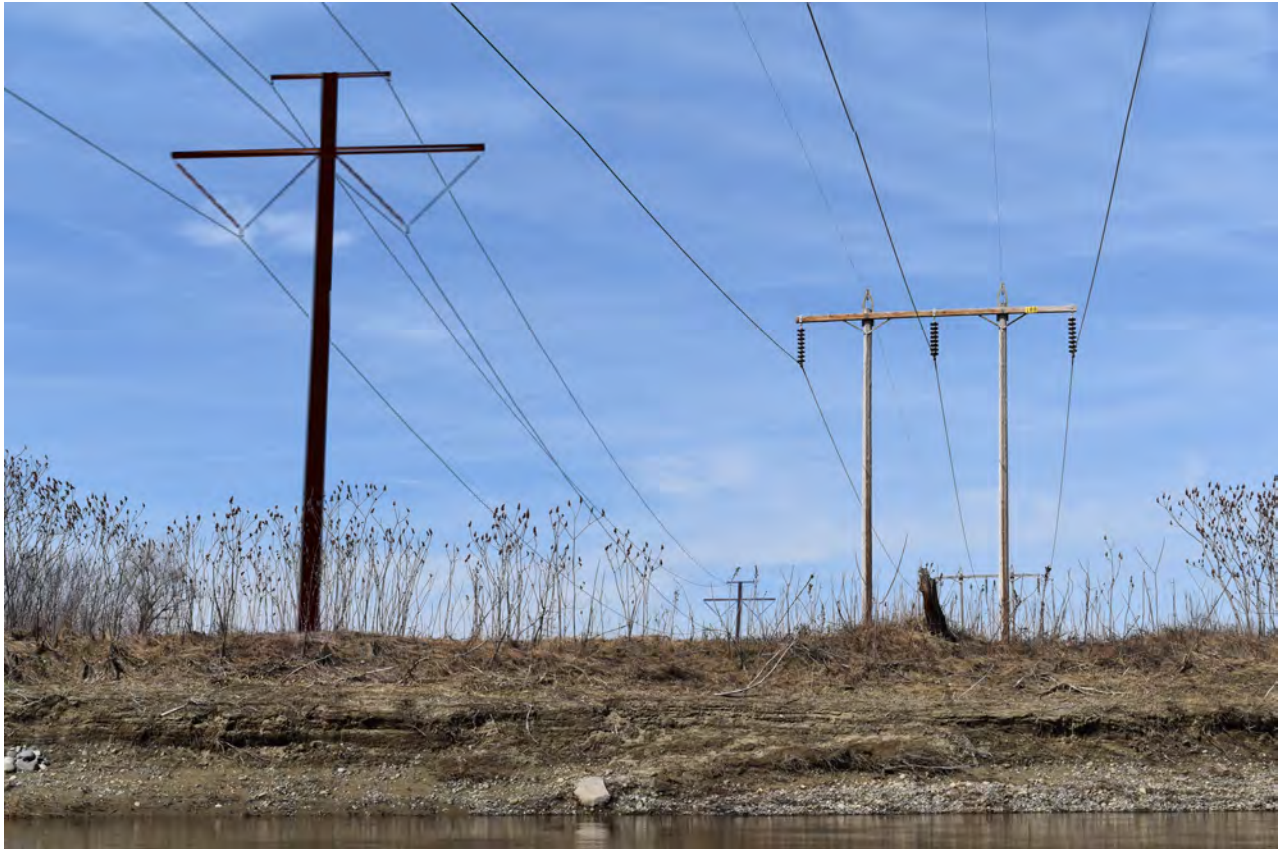
Computer model simulation looking north from Sandy River in Farmington. The closest visible HVDC structure (85 ft in height) would be approximately 150 ft from the edge of the river. No additional vegetation removal would be necessary on the northern edge of the river.
