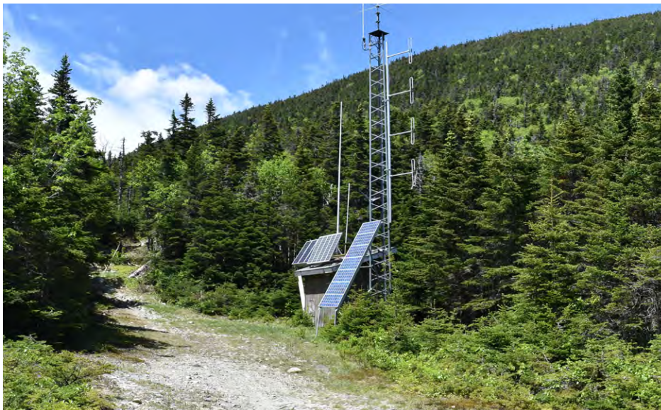
Photograph 8: View looking northwest of communication structures in the cleared area mid-way up Coburn Mountain.
