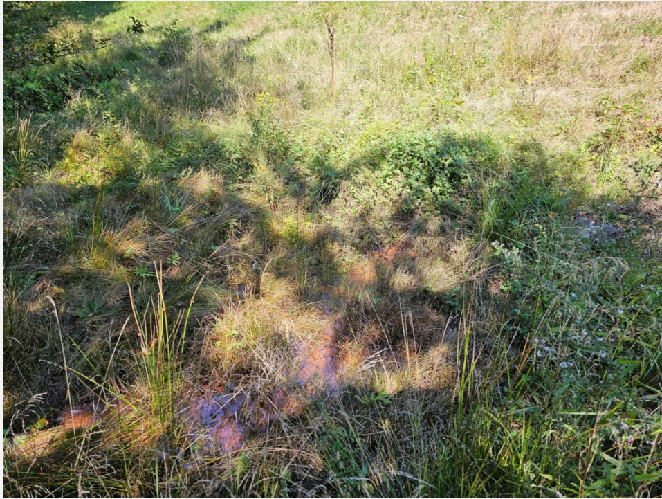
Photo 3 – Earthen Dam Downstream Base Seep East Side
