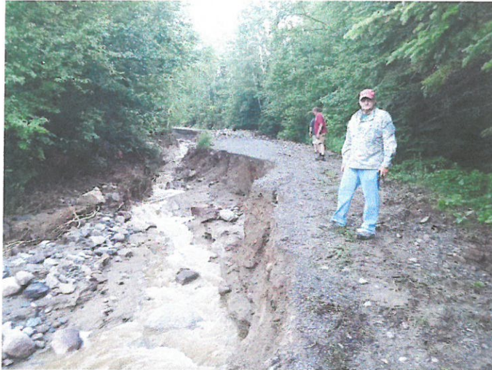
State Rep. Larry Dunphy, of Embden, stands by a washed-out road in northwestern Somerset County Wednesday. Dunphy said he is trying to help secure financial help for residents of the area to fix the damage, which is estimated to be hundreds of thousands of dollars. Contributed photo (Waterville Sentinel July 1, 2016).
