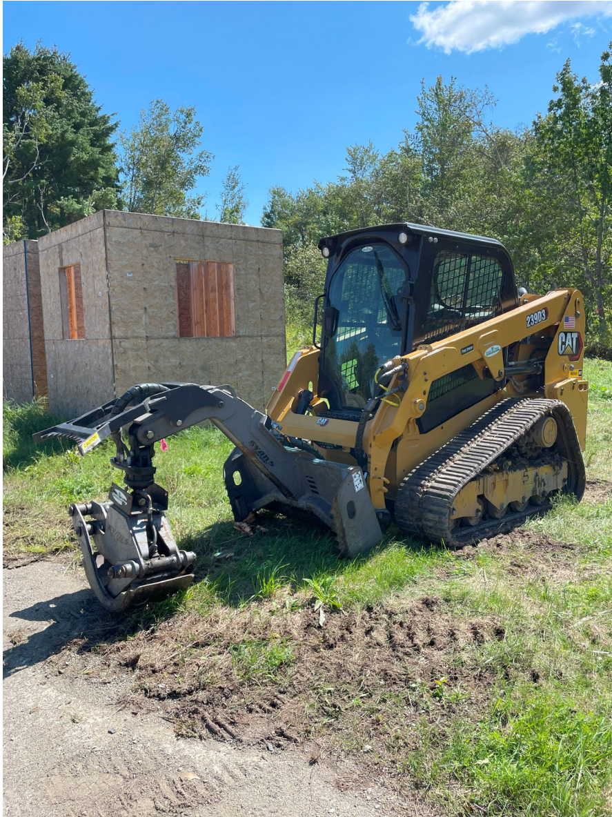
PHOTO 003: Skid steer equipped with log grabber. Machine was used to position logs over wet areas to allow sonic drill rig to traverse without leaving ruts in the soil.
