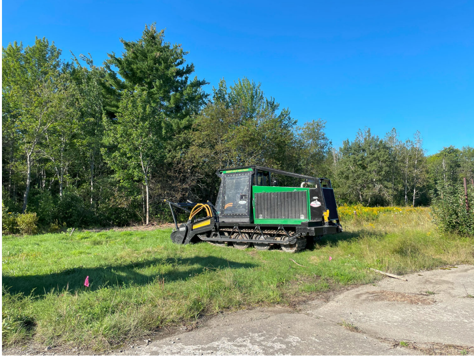
PHOTO 001: Forestry brush hogger. Trails were marked out and cleared to avoid removing trees with limb diameters greater than 3"
