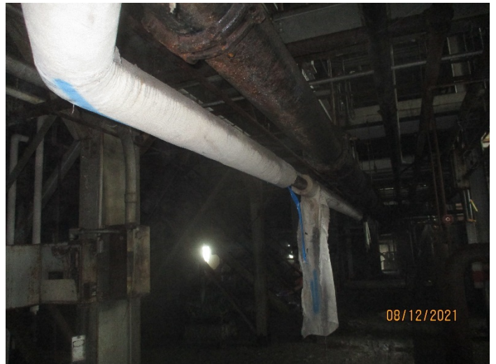
Photo 1&2-26: Non-ACM by Analysis
