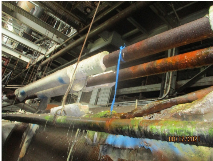
Photo 1&2-31: Non-ACM by Analysis
