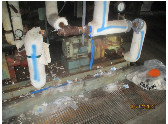
Photo 1&2-10/11: Non-ACM by Analysis
