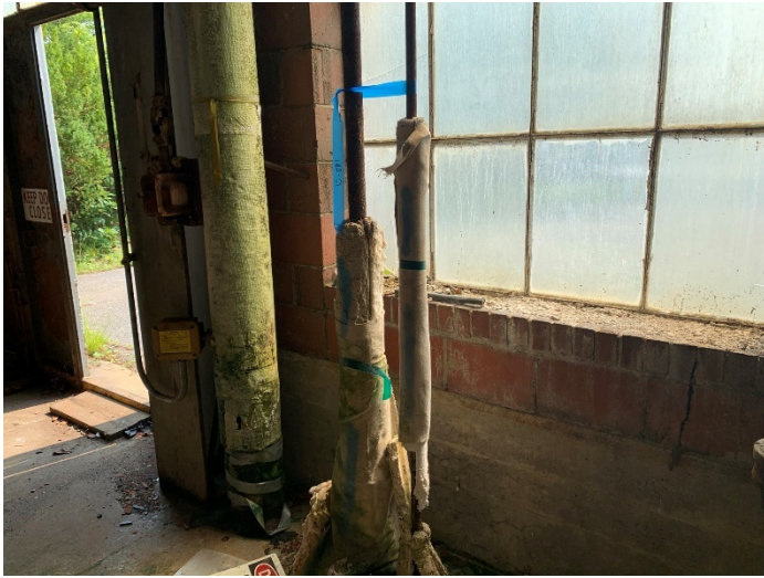
Photo 1&2-01: Non-ACM by analysis
