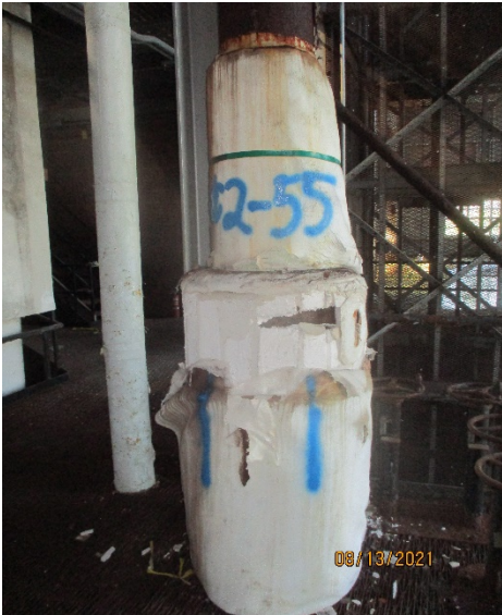
Photo 1&2-55: Non-ACM by Analysis
