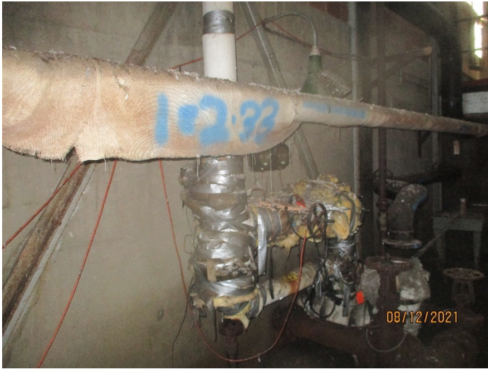
Photo 1&2-33: Non-ACM by Analysis
