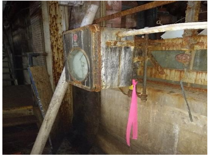
Location M08: Bailey Meter, no tag indicating if it has been drained.
