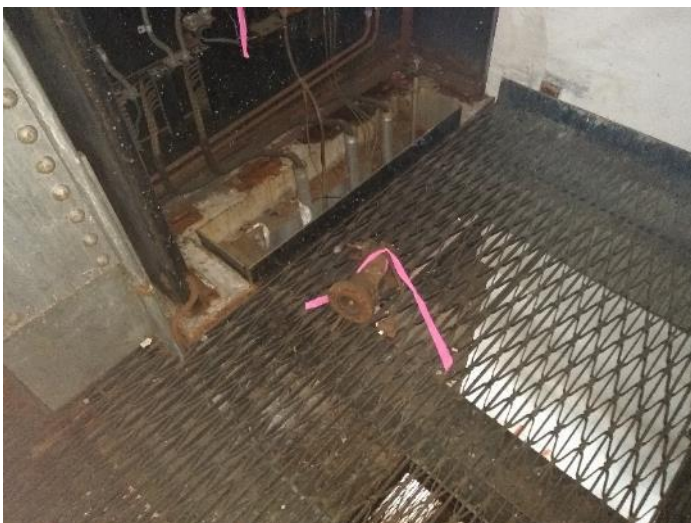
Location M17: View of reservoir formerly containing mercury situated on the floor.
