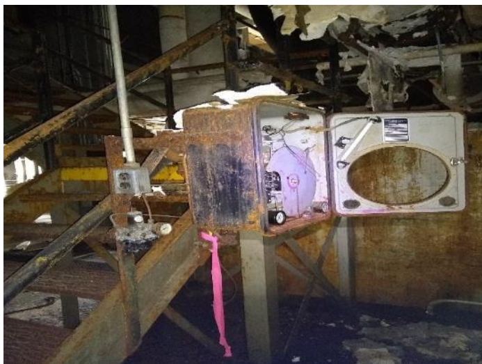
Location M05: Bailey Meter, no tag indicating if it has been drained.
