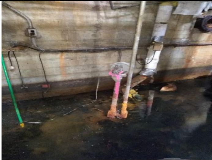
Location M01: View of two mercury ampoules located on a float switch in the basement towards the north portion of the powerhouse.
