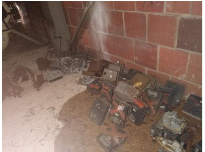
Location M20: Various Bailey Meters and other equipment that formerly or currently contain mercury.
