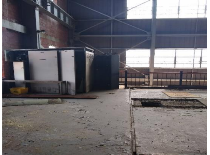
Location M15: View of equipment lockers located to the west of former #7 Boiler.
