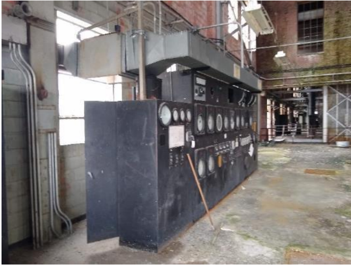
Location M14: View of equipment lockers located to the west of former #7 Boiler.
