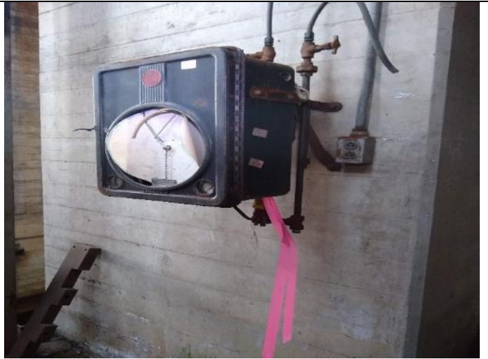
Location M02: View of Bailey meter located to the north portion on the ground level.
