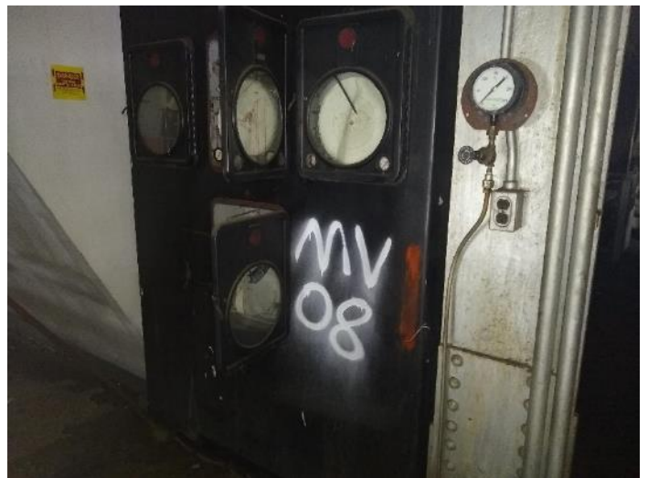
Location M17: View of equipment locker situated between the #5 and #6 boilers on the third level.
