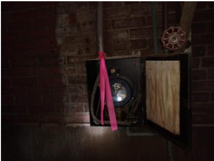
Location M09: Two Mercoïd® switches with the ampoules still in place.
