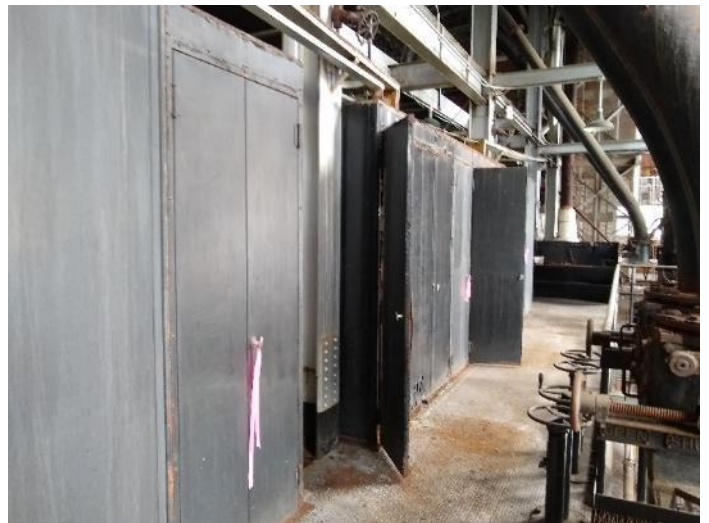
Location M13: View of equipment lockers located to the west of the #1 and #2 boilers.
