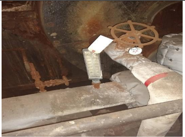
Location M19: Mercury thermometer attached to piping on mezzanine between 2 nd and 3 rd floors.
