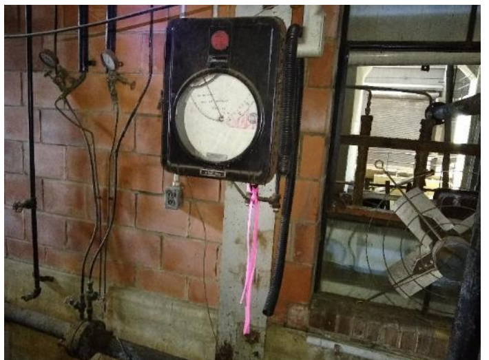
Location M06: Bailey Meter, no tag indicating if it has been drained.
