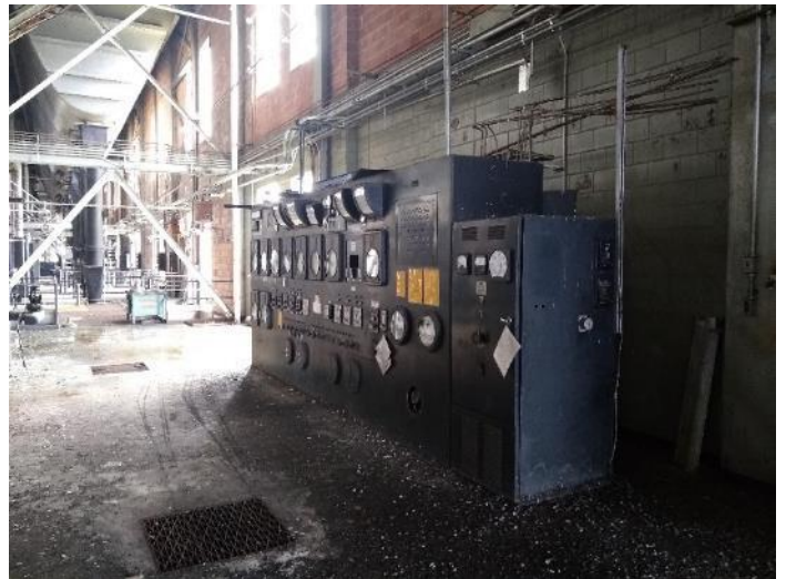
Location M10 & M11: View of equipment locker located in the northwest portion of the building.
