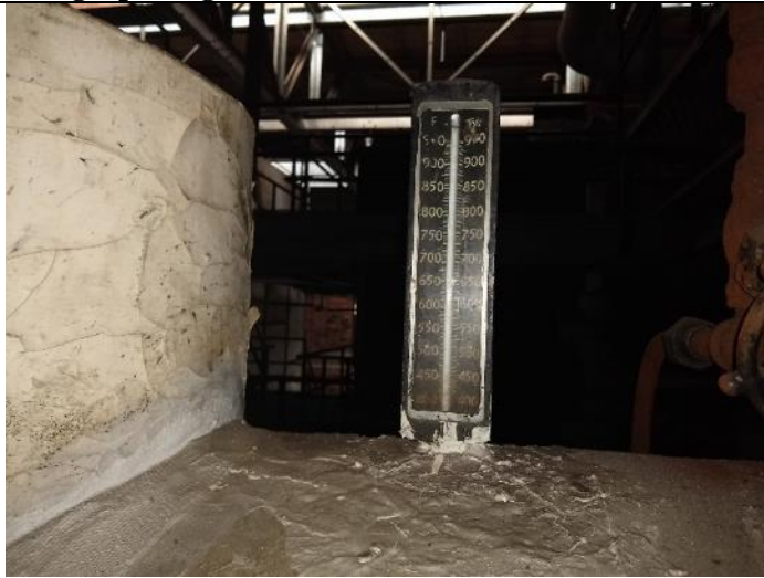
Location M18: Mercury thermometer attached to #4 boiler.
