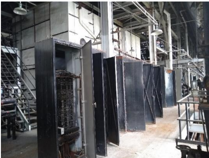
Location M12: View of equipment lockers located to the west of the #3 and #4 boilers.
