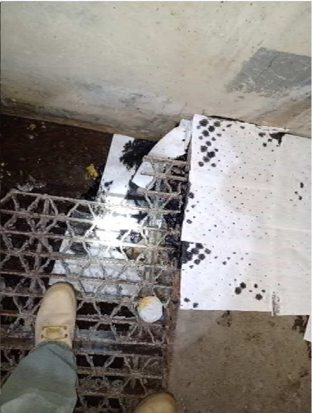
Photo 15: #6 oil from release overhead pipe in floor trench. first floor, Unit 5.
