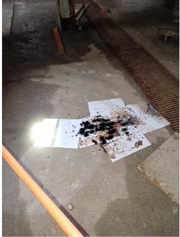
Photo 9: #6 oil release from equipment locker. First floor, Units 1 & 2.
