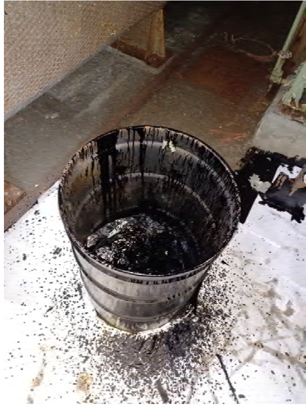
Photo 13: #6 oil release from equipment locker. First floor, Units 1 & 2
