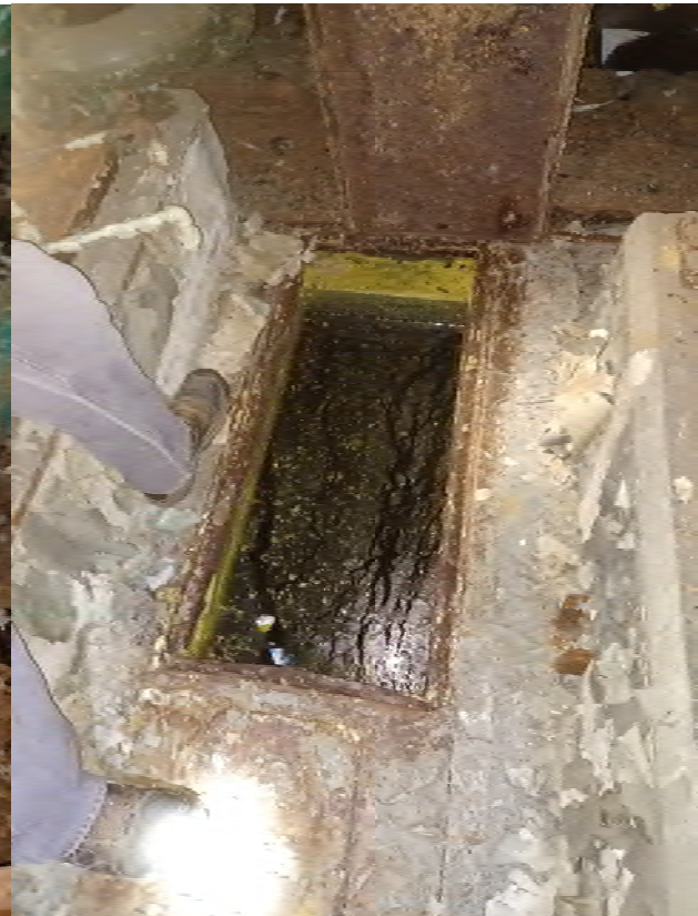
Photo 19: Unknown yellow oil release in floor vault and trenches. First floor, Units 1 & 2.
