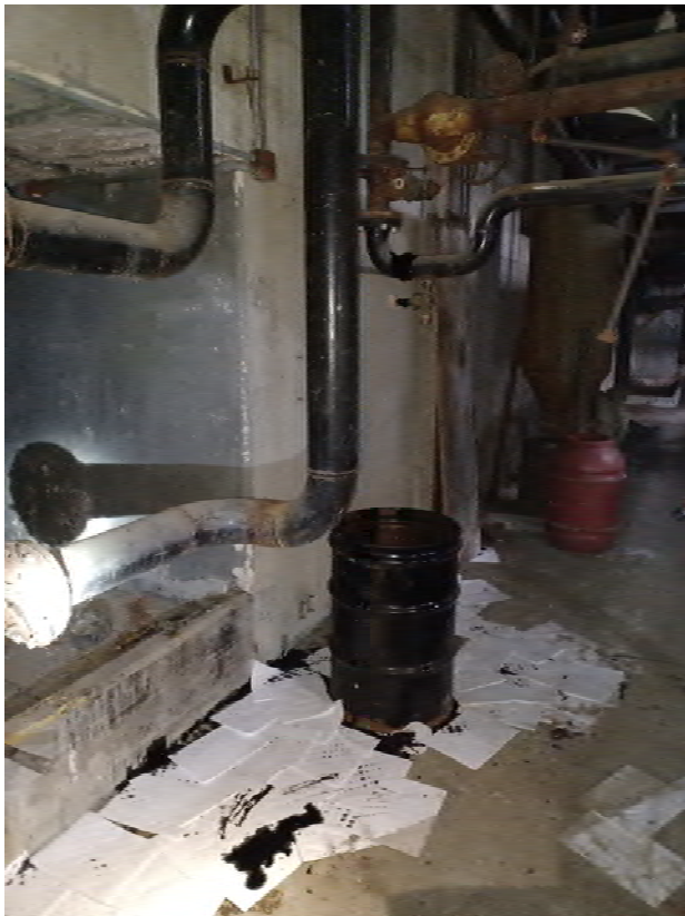
Photo 14: #6 oil release from leaking overhead pipe first floor, Unit 5
