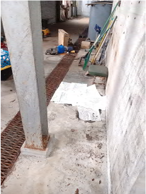
Photo 4: Roofing tar release, 1 st floor, Units 3 & 4
