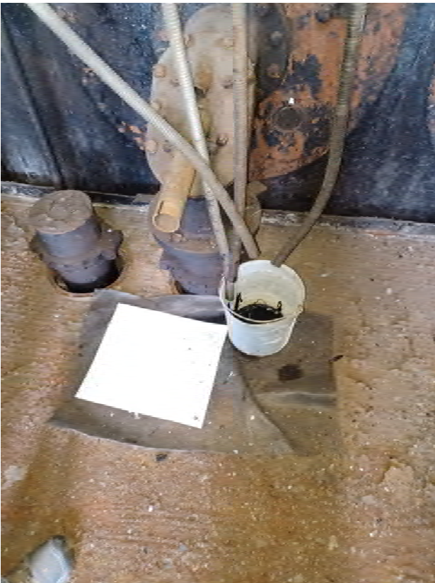
Photo 23: Severed pipes from boiler on third floor, Units 1 & 2.
