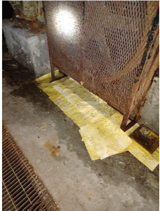
Photo 5 : Unknown yellow oil discharging from series of pumps. 1 st floor, Units 3 & 4.
