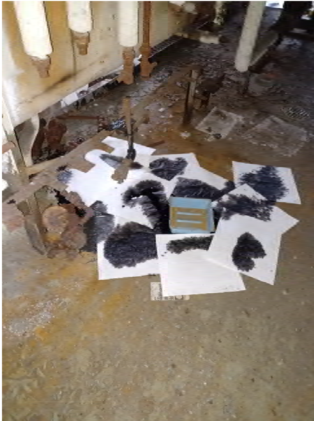
Photo 20: Release of #6 oil from heater bank on 2 nd floor, Units 3 & 4.
