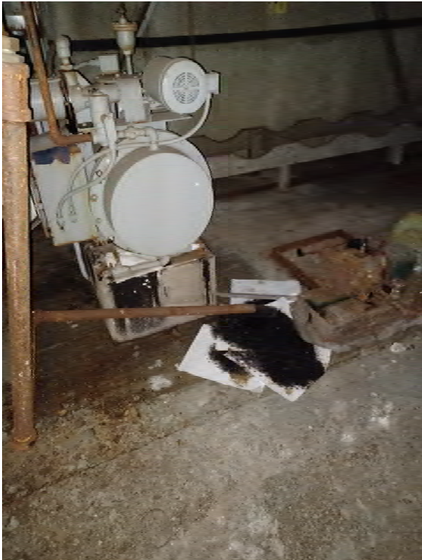
Photo 10: #6 oil release from equipment locker. First floor, Units 1 & 2.
