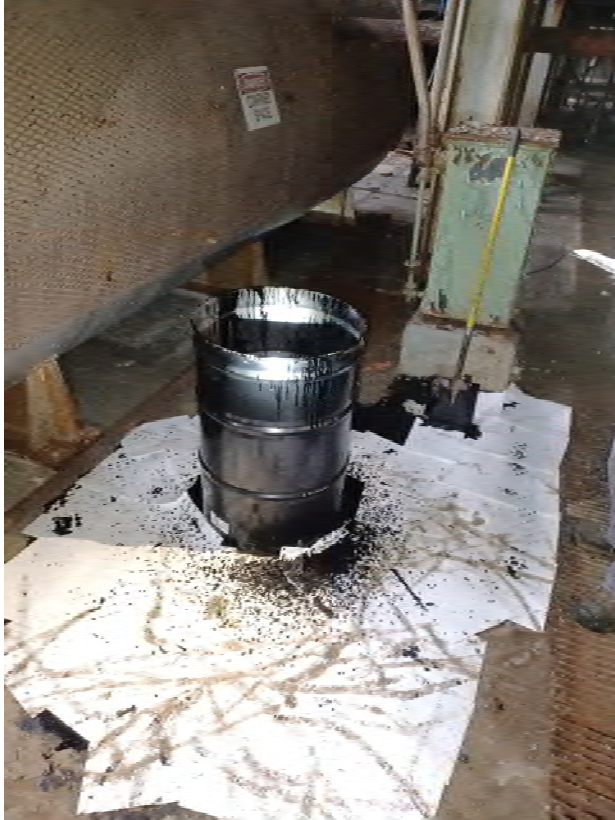
Photo 12: #6 oil release from equipment locker. First floor, Units 1 & 2
