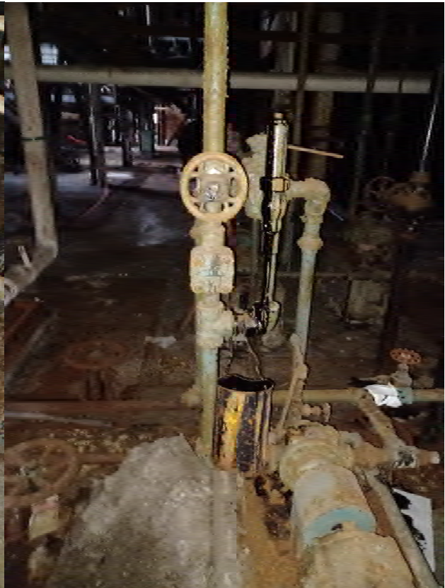
Photo 17: #6 oil release from leaking pipe. First floor, Unit 1 and 2.
