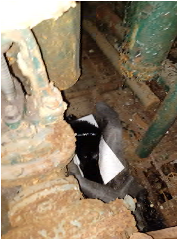
Photo 18: Oil release from leaking pipe. First floor, Unit 1 and 2.
