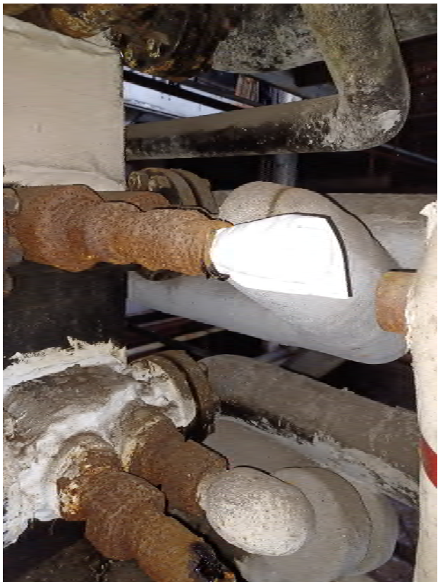
Photo 22: absorbent pad plugging the leak from a heater bank on 2 nd floor, Units 3 & 4.
