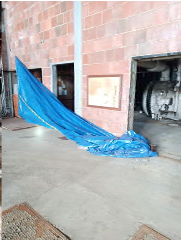
Photo 27: Tarp intended to segregate portion of building and prevent exposure to asbestos has fallen
