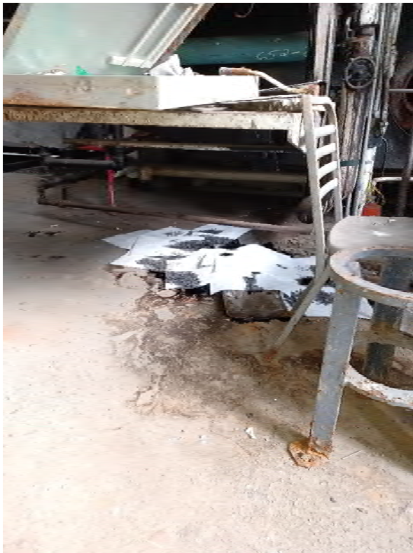
Photo 26: #6 oil release from boiler. First floor, Units 1 & 2
