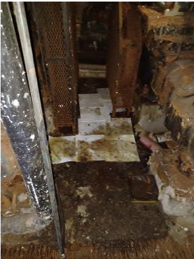
Photo 6 : Unknown yellow oil discharging from series of pumps. 1 st floor, Units 3 & 4
