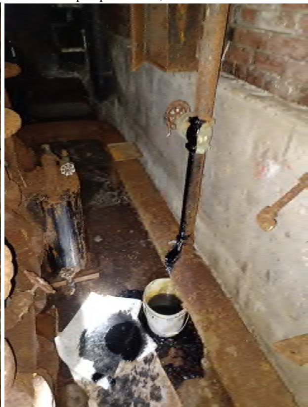
Photo 7: #6 oil release from severed pipe. 1 st floor, Units 3 & 4.
