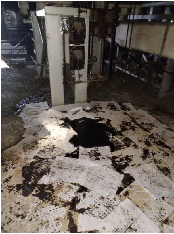
Photo 1: #6 oil release 2 nd floor Units 1 & 2
