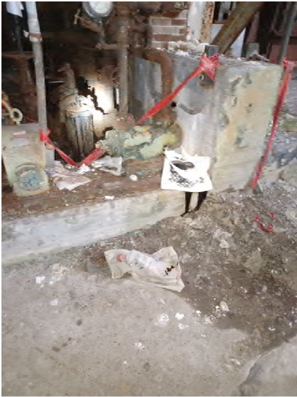
Photo 8: #6 oil release from severed pipe. 1 st floor, Units 3 & 4
