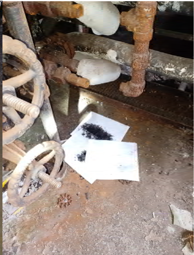
Photo 21: Release of #6 oil from heater bank on 2 nd floor, Units 3 & 4.
