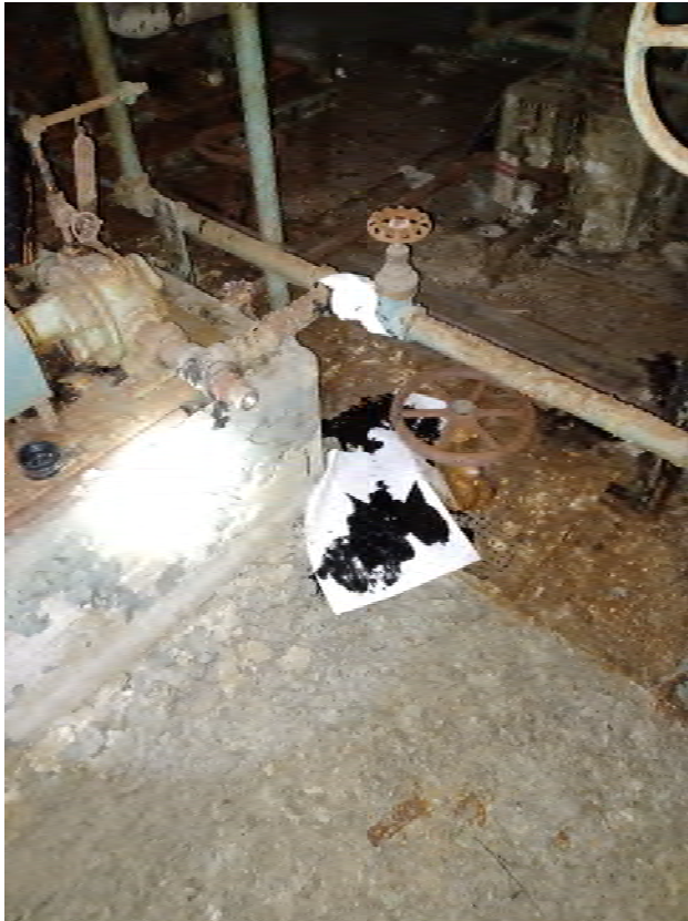
Photo 16: #6 oil release from leaking pipe. First floor, Unit 1 and 2.
