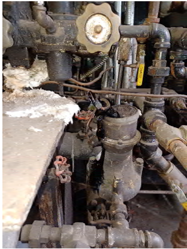
Photo 25: Leaking pipe on boiler. First floor, Units 1 & 2
