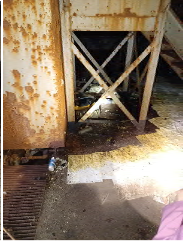
Photo 2: #2 Gearbox oil release, 1 st floor Units 1 & 2
