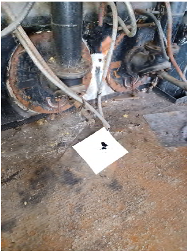
Photo 24: Severed pipes from boiler on third floor, Units 1 & 2.
