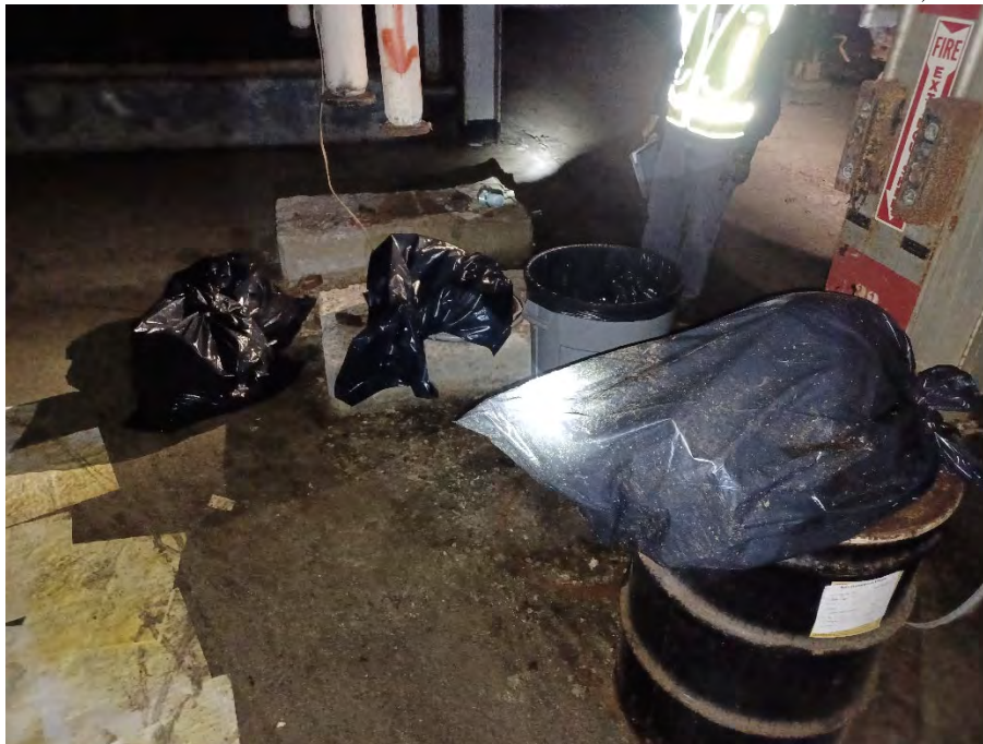
Photo 3: Gearbox oil release, 1 st floor Units 1 & 2 used pads placed in trash bags.
