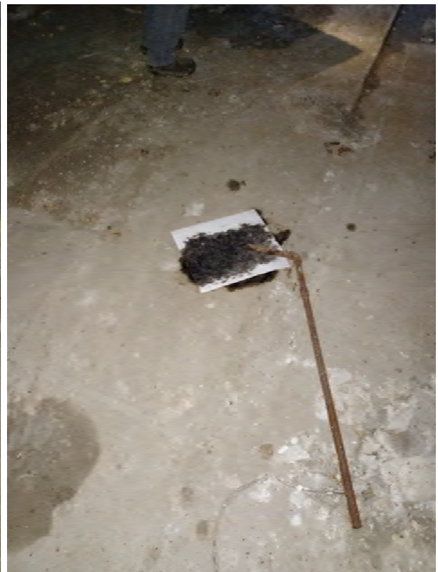
Photo 11: #6 oil release from equipment locker. First floor, Units 1 & 2
