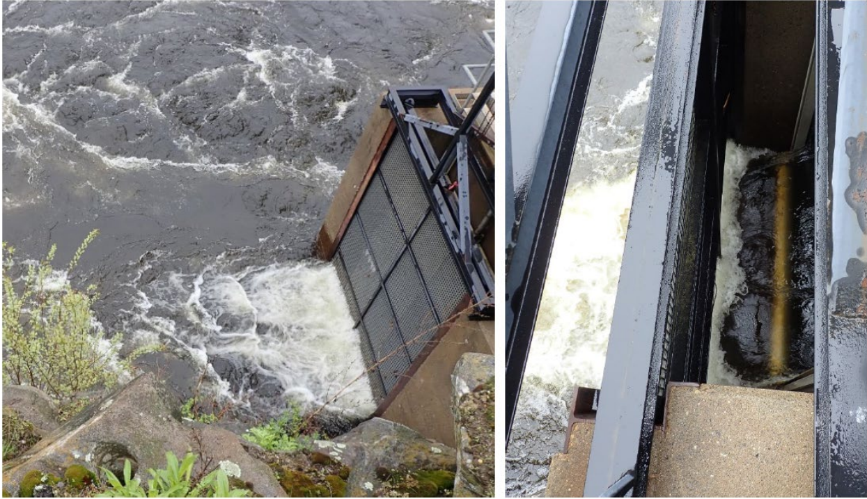
Photograph 1 – Blocking screen submerged in tailwater to skim debris (Left), and entrance gate setting potentially too high (Right)
