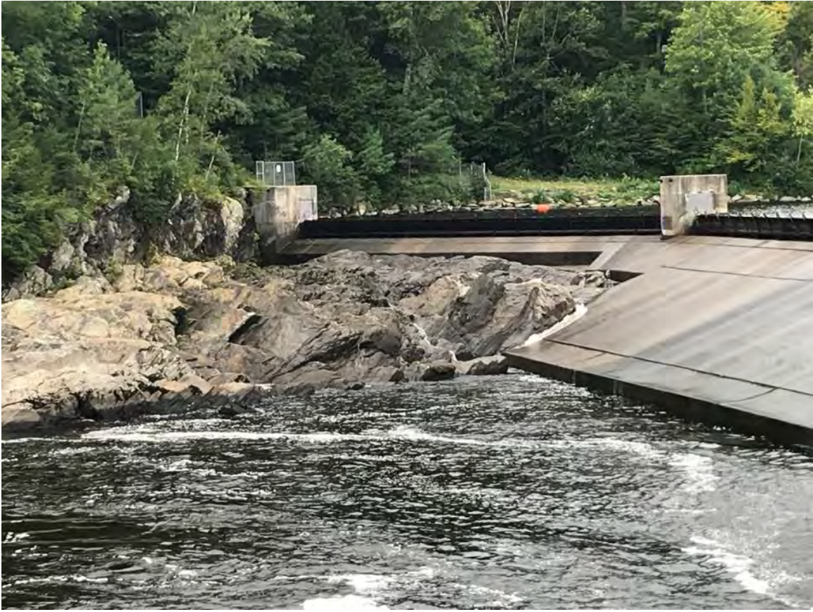
Figure 4.6.1.3.2-3: Exposed Bedrock Area below Bascule Gate No. 5 as Viewed from River Left
