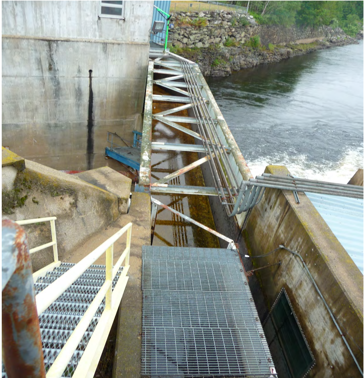
Figure 2.1.3.1-1: Upstream Fish Passage Facility
