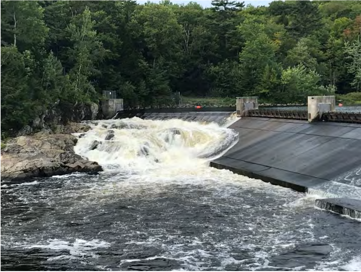
Figure 4.6.1.3.2-2: Bascule Gate No. 5 in Fully Lowered Position
