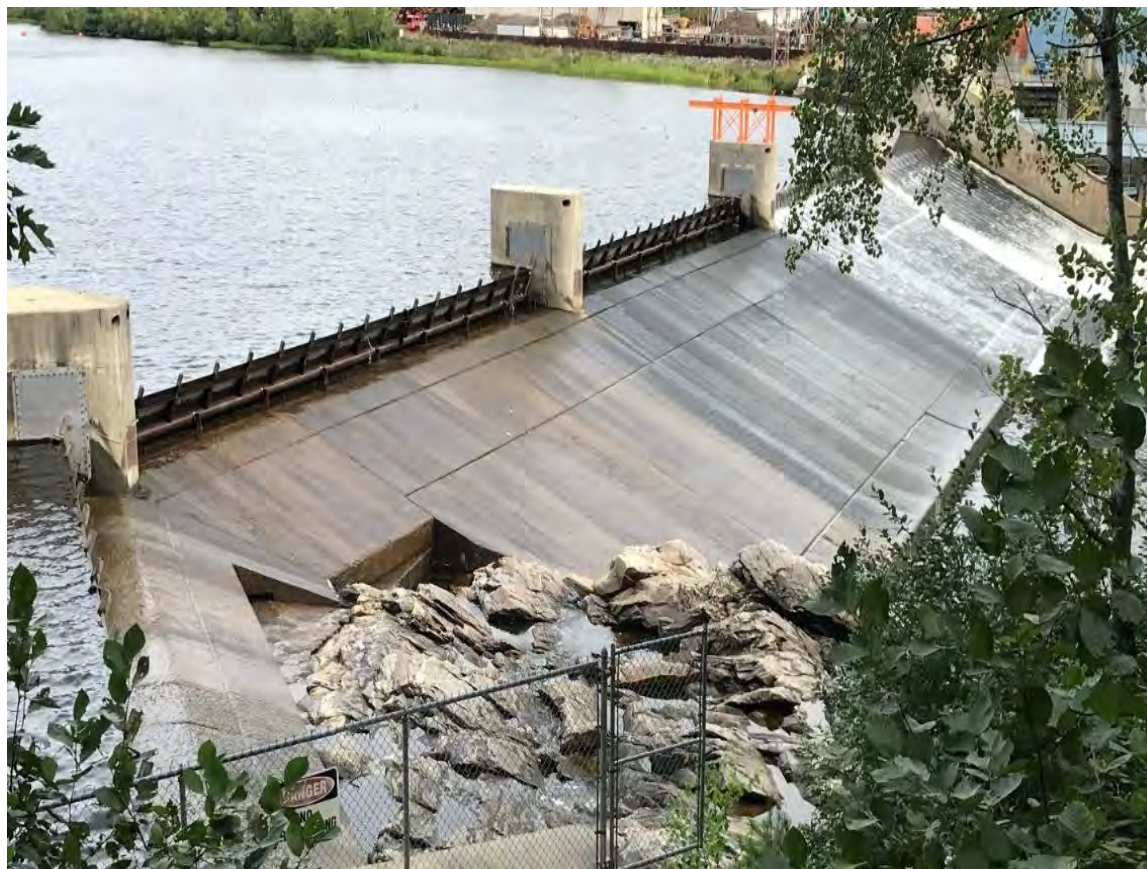
Figure 4.6.1.3.2-4: Exposed Bedrock Area below Bascule Gate No. 5 as Viewed from River Right
