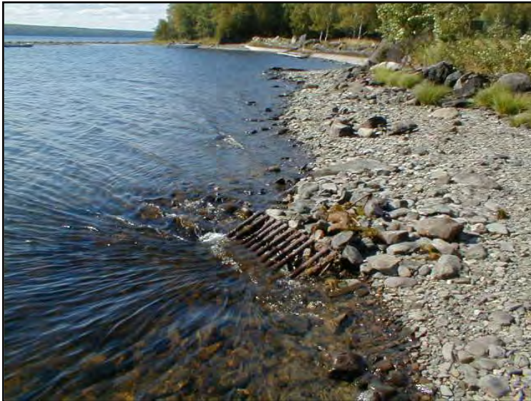
(Left) The Grate and Culvert Enabling Water to Pass through Earthen Lock Dam. Note, photo represents low lake level. (2002 Photo)
