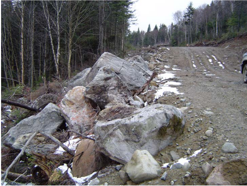
Photo 9: Large boulders utilized on downslope side of fill extension for fill retention and rip rap armament. Photograph by Albert Frick, 11/12/2003.
