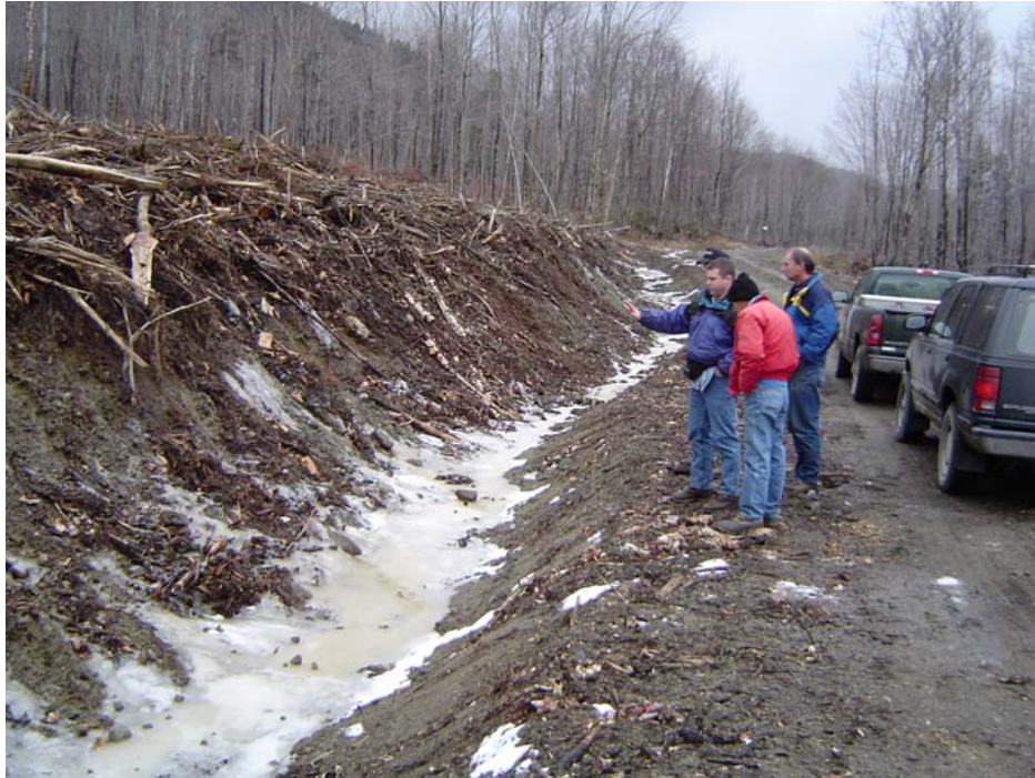
Photo 7: Recently built existing road cut across moderately well drained soil exhibiting seepage on top of soil underlying glacial till. Erosion and sediment control not yet in place. Photographed by A.F. 11/12/2003.
