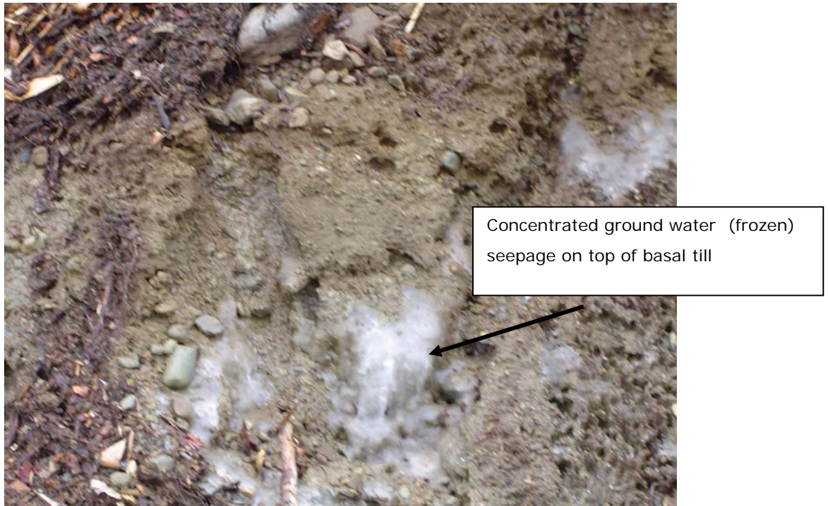
Photo 4: Typical major ground water seep area encountered in mountainous road cut. Photograph by Albert Frick, 11/12/2003.
