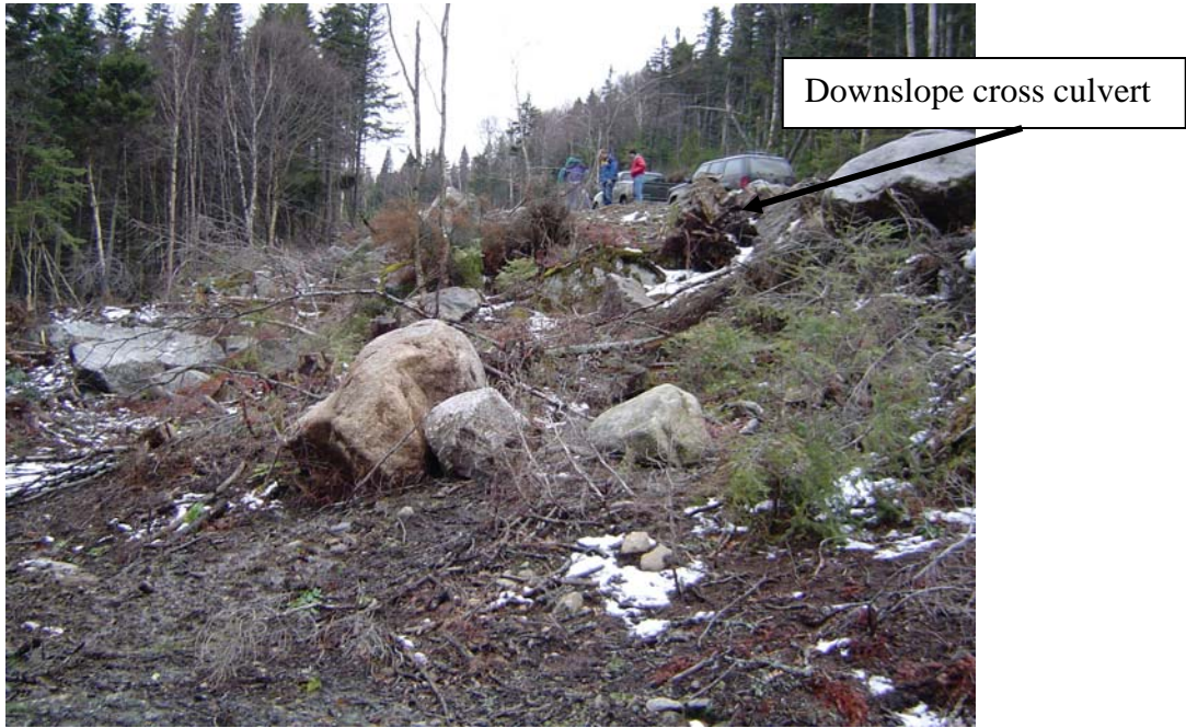
Photo 6A: Downslope cross culvert with stabilized channel utilizing vegetation. Photograph by Albert Frick, 11/12/2003.
